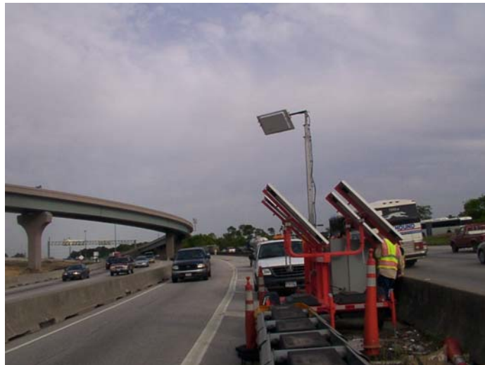
Figure 25. AVI Enforcement Reader at Katy Eastern Extension – AM Direction
